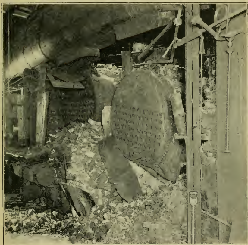
After dairy boiler bulged and ruptured
